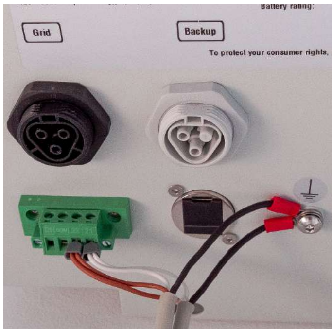
Fig. 60 RS485 connection for master and 1st slave storage unit in a network of 3 SAX Power Home (Plus)
