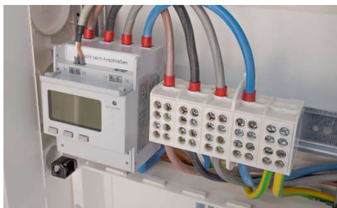
Fig. 36 ADL400 correctly connected
